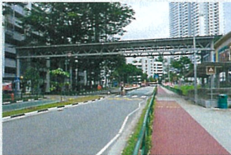
Construction of Low and High Linkway over Pedestrian Crossing from Blk(s) 21 to 14A Lorong 7 Toa Payoh
