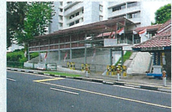
Construction of Low Linkway from existing shelter over BFA Ramp near Blk(s) 25 Sin Ming Road to Bus Stop
