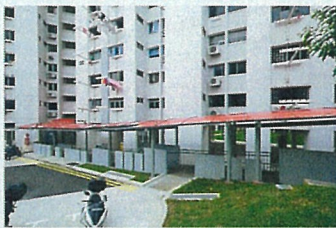
Construction of Shelter over Existing BFA Ramp near Blk(s) 403 Sin Ming Avenue
