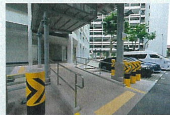
Construction of BFA Ramp at Existing High Linkway at Blk(s) 301 Shunfu Road
