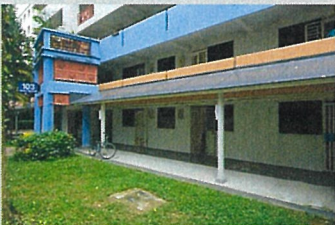
Construction of Fixed Awning at Ground Floor Corridor of Blk(s) 103 Lorong 1 Toa Payoh
